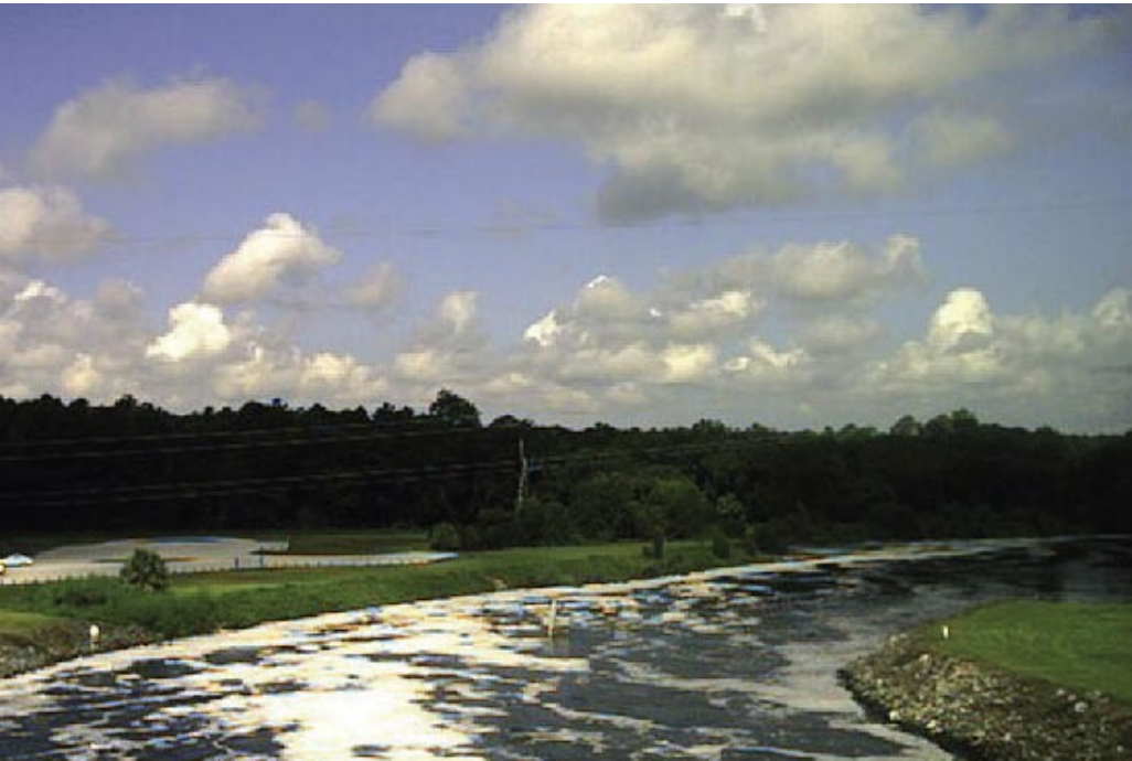
The SFWMD takes care of security for canals, pump stations and flood-control structures.
