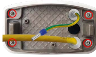
Fig. 12: Installed and ready for Connector Box LSA
