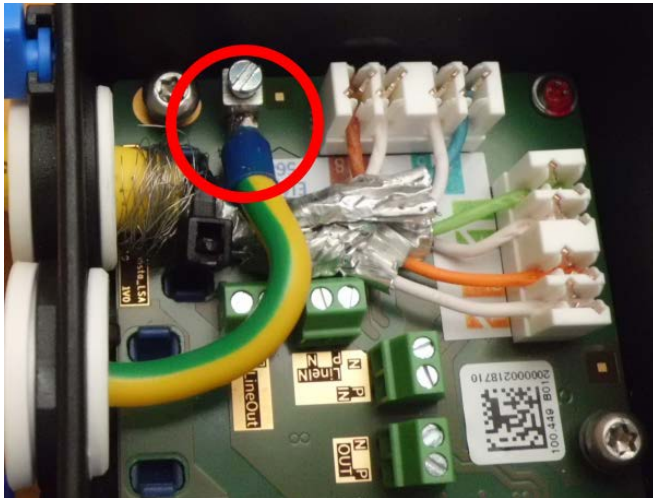
Fig. 30: Ground wire connected to terminal
