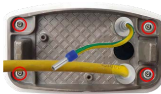
Fig. 7: Installed and ready for Connector Box LSA
