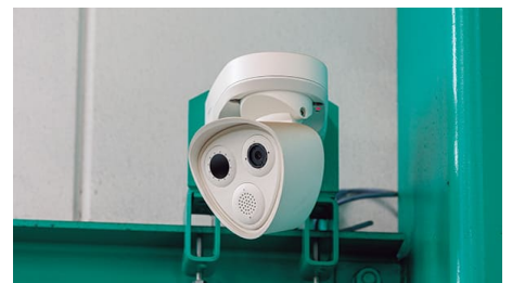
MOBOTIX M73 thermal camera, installed at the collection & sorting facility
